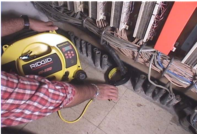
Placing the clamp around the telephone cable helps to isolate it from other lines.
